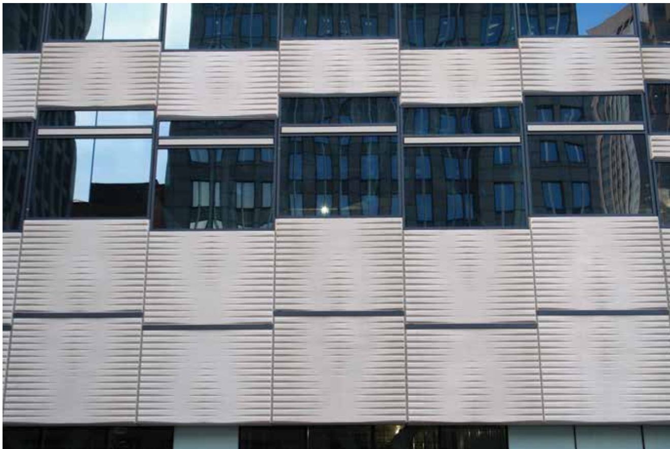
CAD-CAM technology was used to manufacture the master molds for the photo-engraved rose images used on the precast concrete panels cladding the Cleveland Medical Mart & Convention Center. Photo: Architectural Polymers.
